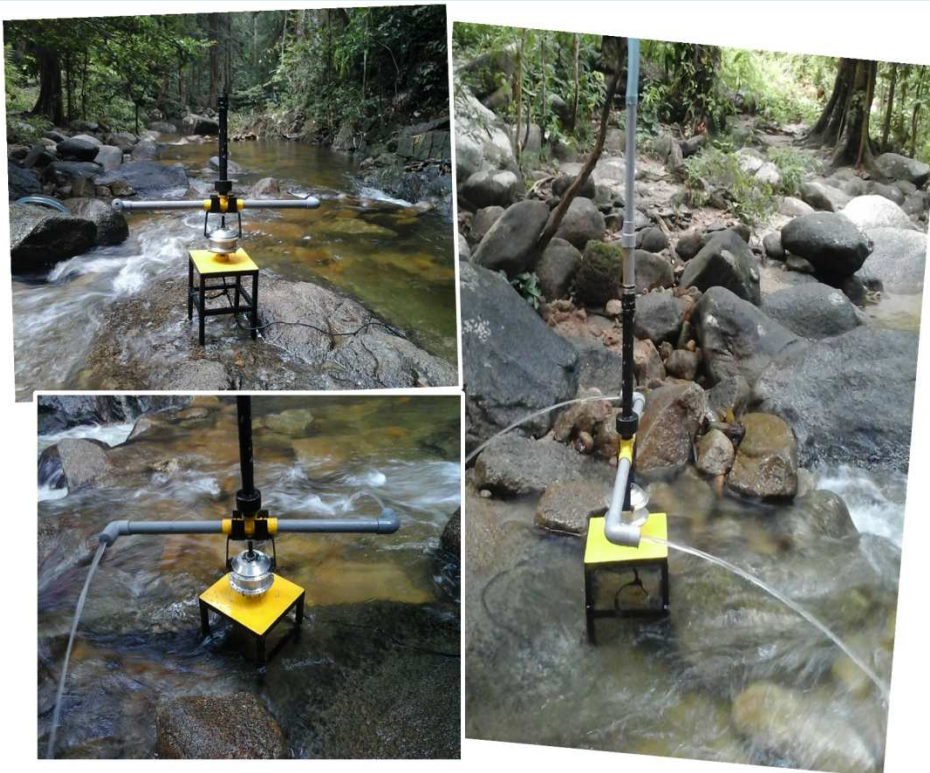
Fig 1 – Pico-hydro generation system at small stream
